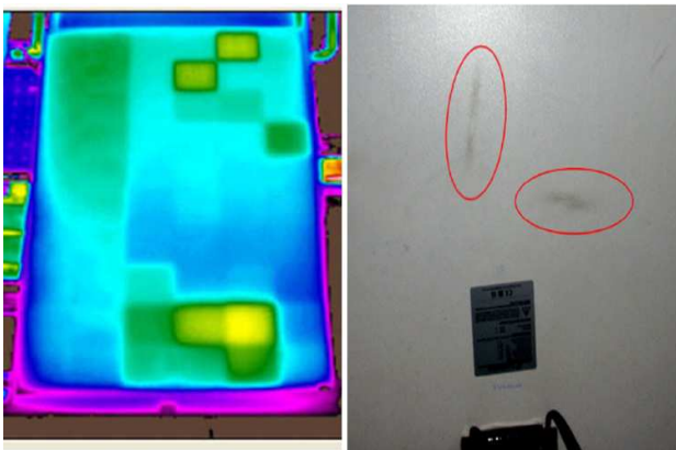
Fig. 5. Sample thermograph and picture of a panel malfunction.
