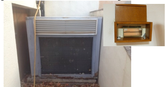
Fig. 1. Old Heat Pump and control system
