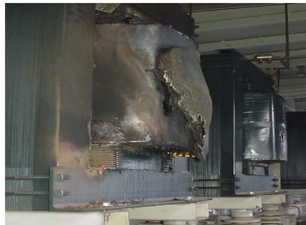
Figure 5. Failed iron core reactor.
