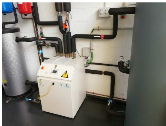
Fig. 8. The module of geothermal energy
