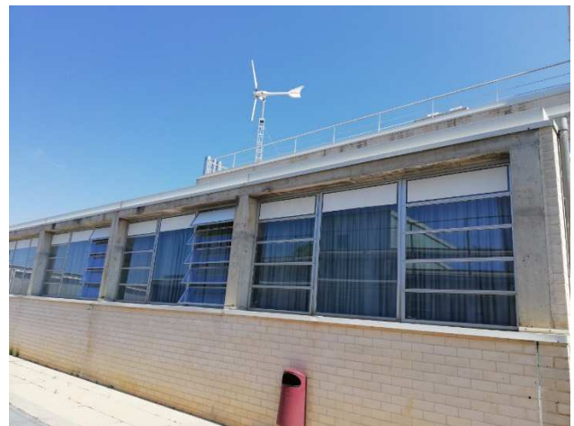
Fig. 3. Mini-wind turbine placed at the roof of P2.
