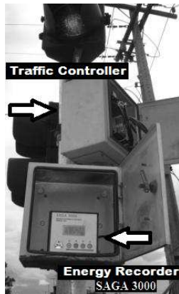
Fig. 3. Measurements made at pedestrian lights with incandescent lamps before replacing.
