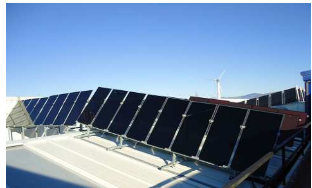
Fig. 3 Isolated photovoltaic system on the FHa roof
