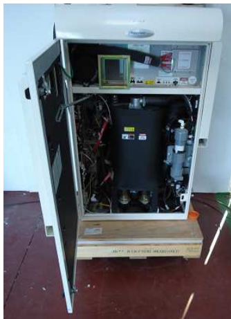
Fig. 4. 5kW fuel cell
