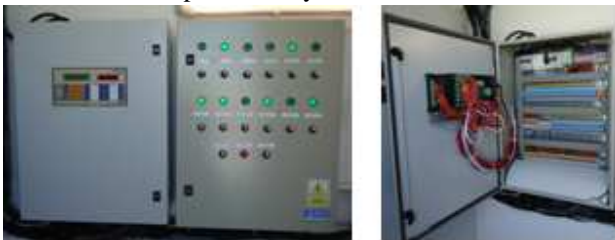
Fig. 9 Electrical panel and programmable automaton Furthermore, a web application has been developed in order to do an on-line control. It is possible to observe the
