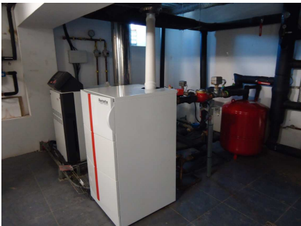
Fig. 8 Heating boilers and its integration with the solar thermal system inside the boilers room.
