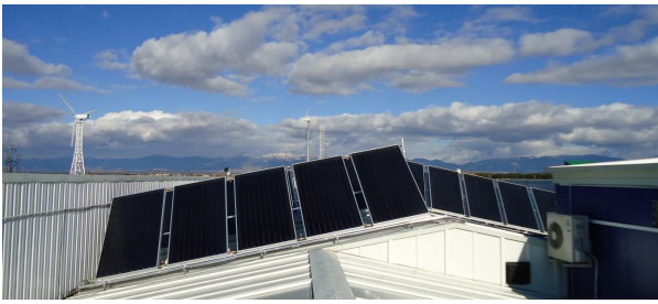
Fig. 7 Solar thermal system on the roof of the FHa building.
