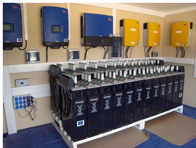
Fig. 5. View of the inverters and batteries.
