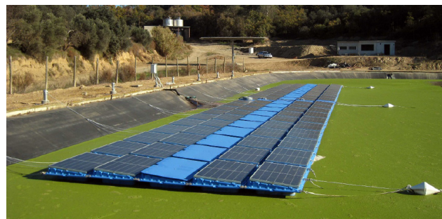
Fig. 3. View of the floating PV installation
