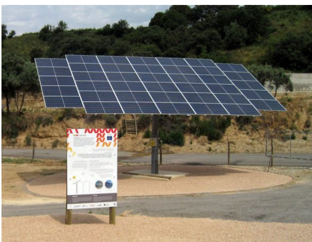
Fig. 7. View of the PV installation with solar tracker (two axes).
