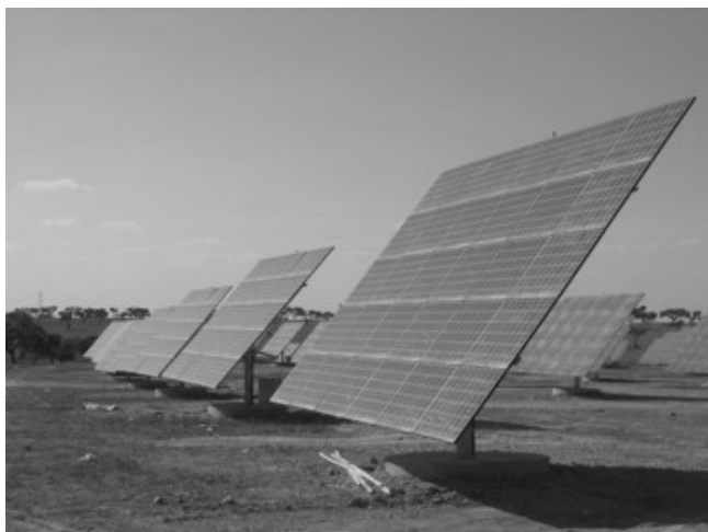
Fig. 4. Solar Park – PV panels
