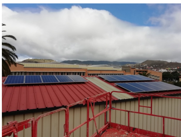
Fig.2. Aerial view of the photovoltaic installation.
